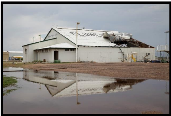
The damage to the Qantas hangar at the Cloncurry Airport in January 2014.
